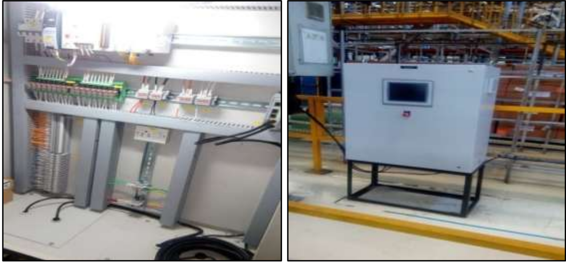
Figure 4.26: Internal and external view of main PLC
