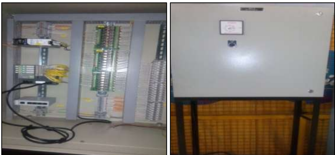
Figure 4.27: Internal and external view of remote I/O panel of PLC
