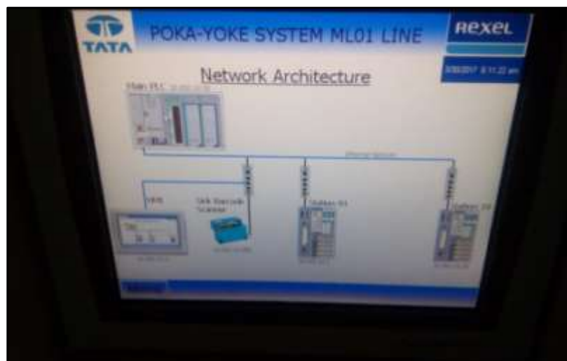
Figure 4.30: Display of network architecture on HMI screen
