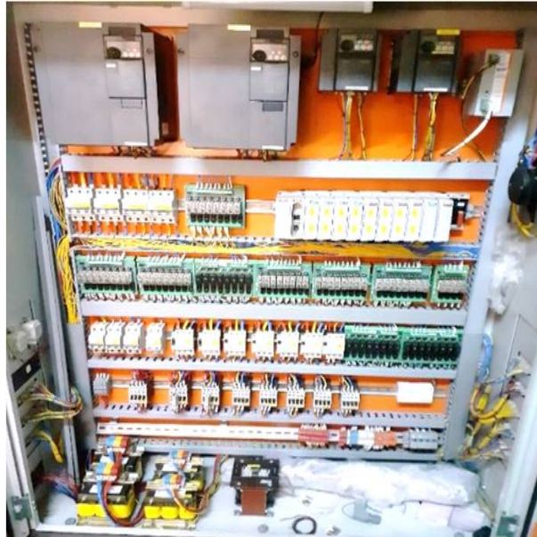
Figure 4.10: PLC controlled panel with VFD control for special purpose machine (SPM)
